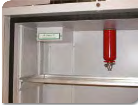
Fire-extinguisher installed in a safety cabinet
